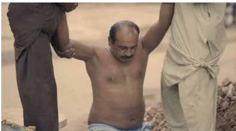
1A WASA Sanitation Worker being lifted into a sewer for cleaning purposes with no safety or protective equipment. (Source: PWF)
